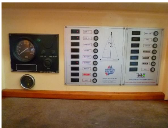
Unadulterated, original switch panels
