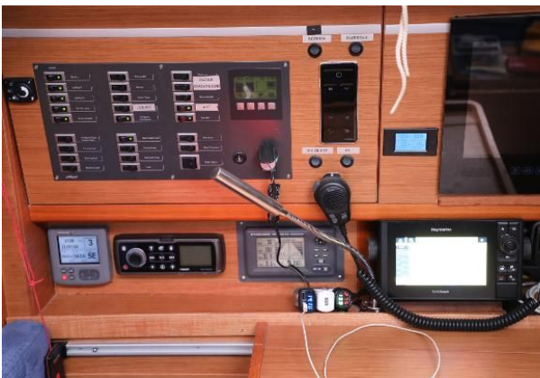
Detail of main 12V DC distribution panel
